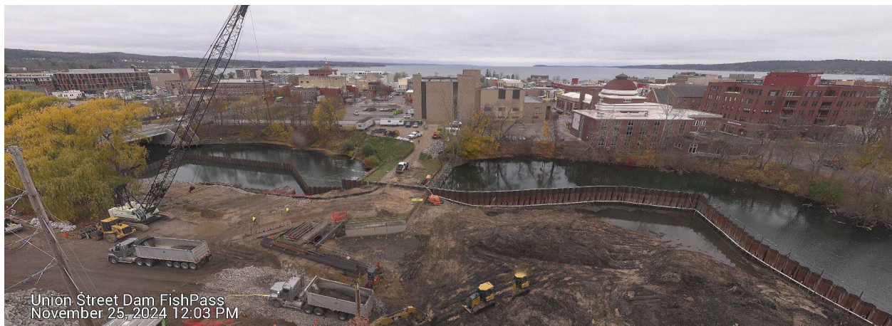
Figure 1. Image captured from the FishPass time-lapse camera: November 25, 2024 – 12:00 PM showing the completed installation of the sheet pile cofferdam upstream (right side of image) and downstream of the dam (left side of image).
